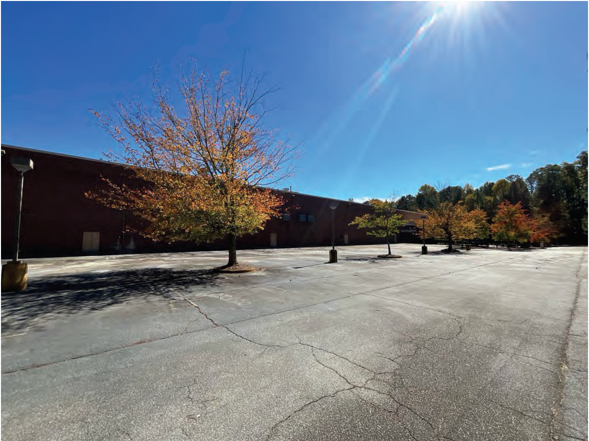
Parking lot trees are fair to Poor condition
