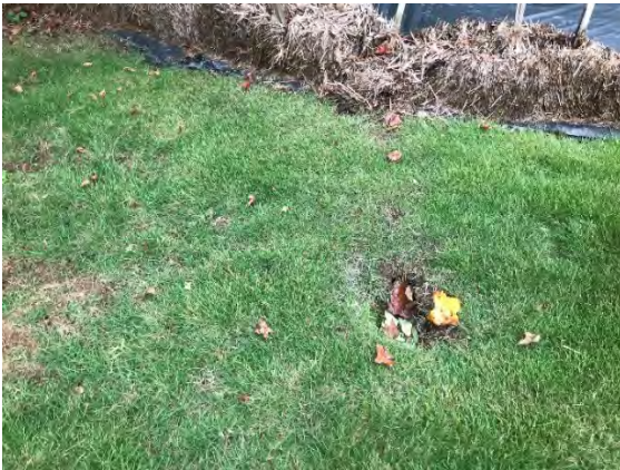
Picture 3: Sinkhole In Backyard
