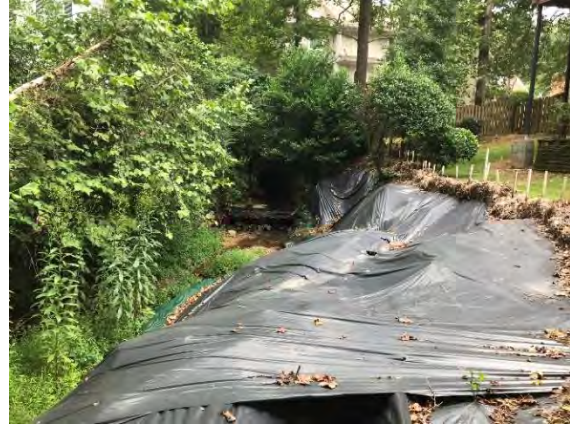
Picture 2: Eroded Streambank
