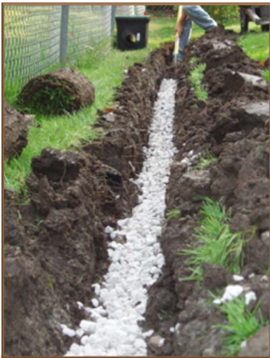
A modified French drain should be constructed in a manner to minimize earth disturbance.
