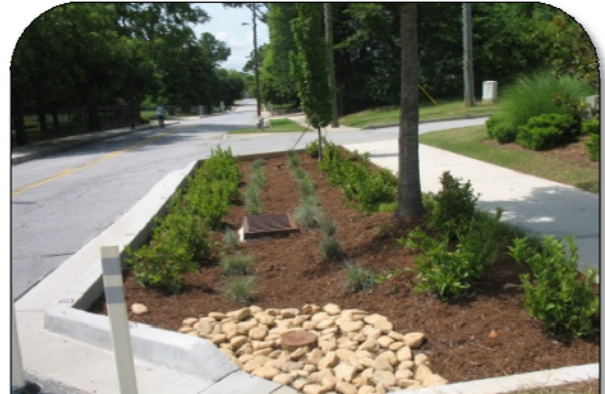
The pretreatment area and overflow structure have been properly maintained and are clear of debris.
