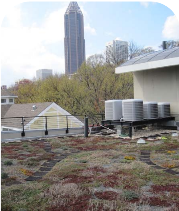
Extensive Green Roof Example. A simple monoculture of sedum with maintenance access provided by rubber walkway stones.
