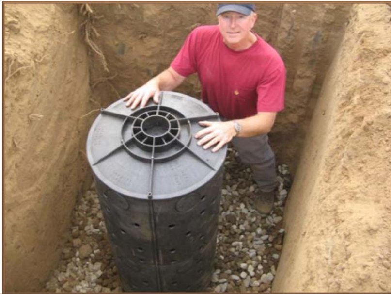
A dry well being placed during construction. Special attention should be placed on ensuring the excavation bottom surface is properly scarified.
