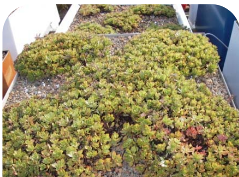
An extensive green roof should reach 90% growth coverage within two years.
